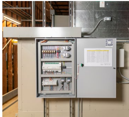
New HVAC controls in place
