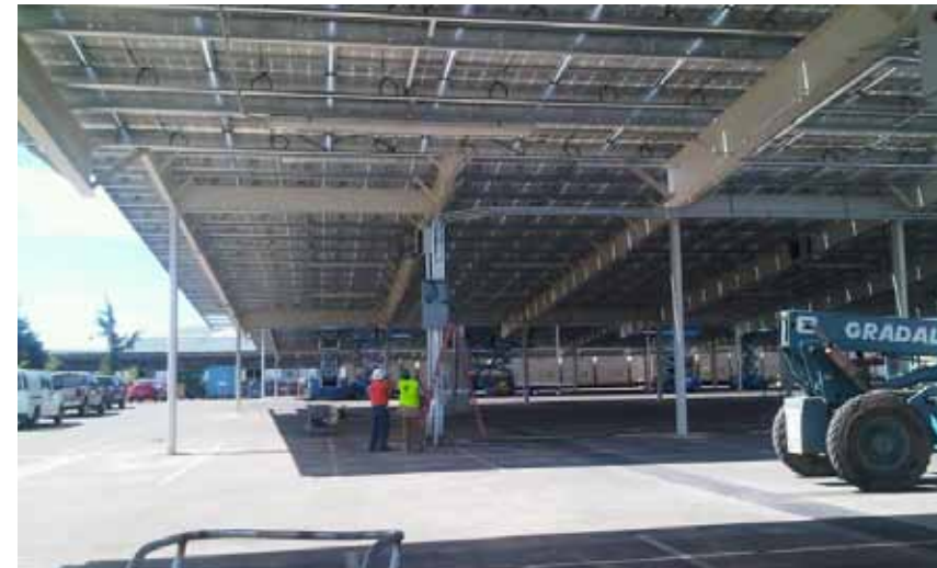
Solar PV covered parking, Siemens Mobility, Sacramento, California
