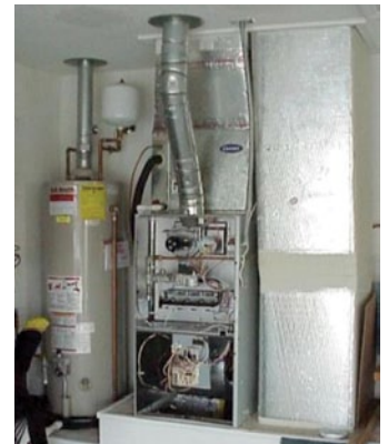
Gas furnace with panel removed. Cabinet and return duct leakage can interfere with natural draft appliances such as the gas water heater at left.
