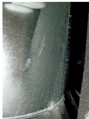
Moisture and watermarks on fan housing.
