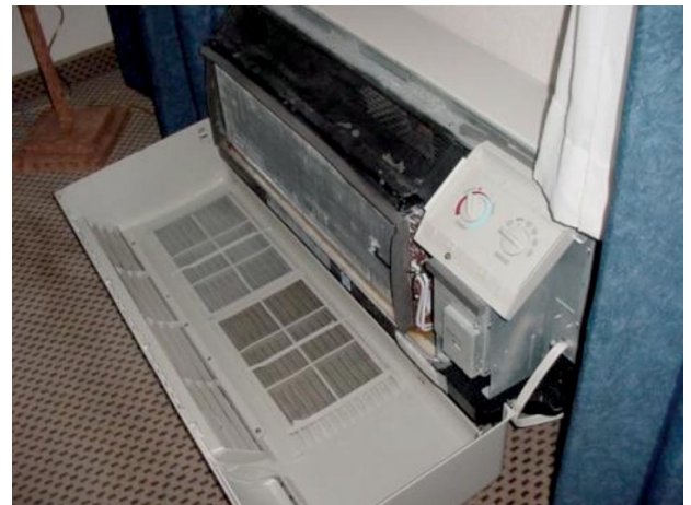
PTAC unit was not tilted toward the drain correctly and water spilled from condensate pan onto carpet below.
