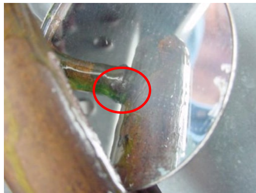
Mirror and dye used to locate leak.
