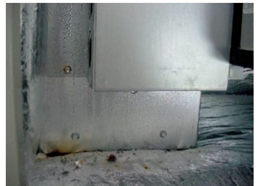
Condensation on metal electric box inside air handler.
