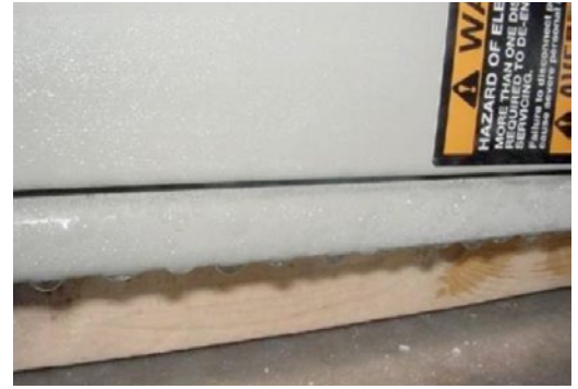
Condensation at bottom of air handler caused by wet interior insulation, rendering the insulation
