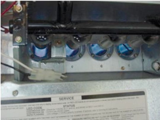
Light blue flames indicate clean efficient combustion.
