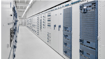
Electrical switching rooms
