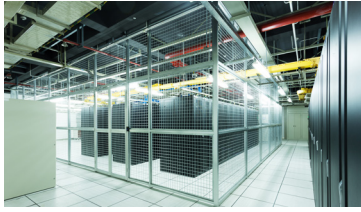
Data centers and server rooms
